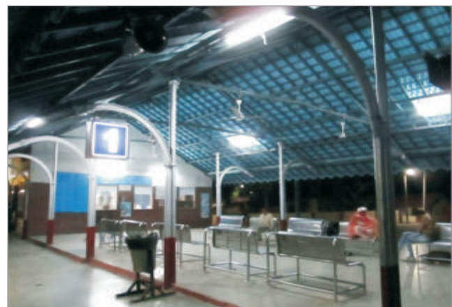
LED lights installed at Railway stations
