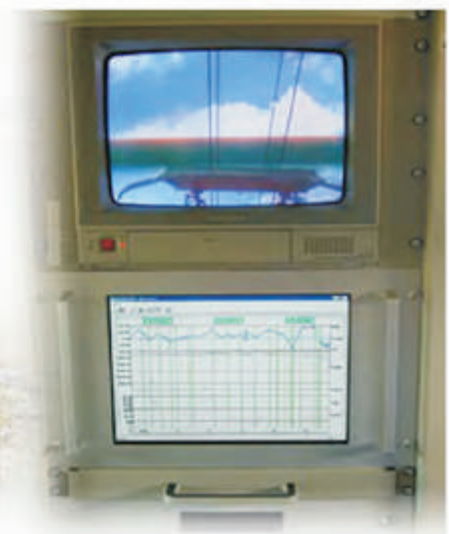
Tower Car with Measuring & Recording Instrumentation (for predictive maintenance)
